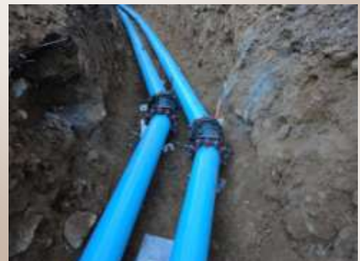
Water Distribution Lines
